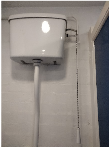
Figure 14: Example of the one -stage toilet tanks in West Block
