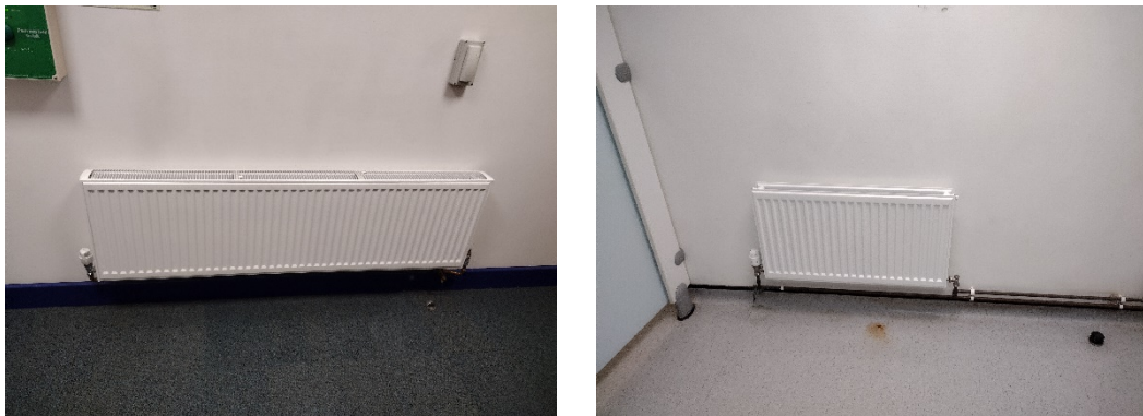
Figure 4: Examples of heating devices in the Robin Brooke Centre
