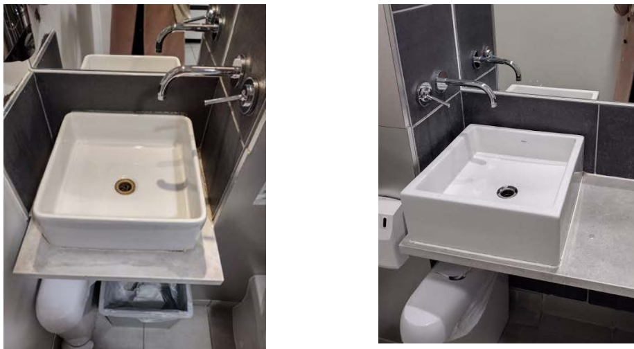
Figure 4: Examples of water mixing taps
