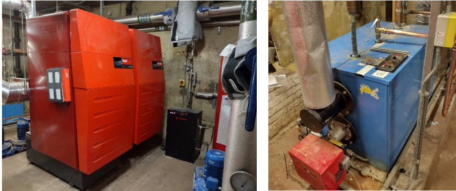
Figure 3: Installed boilers in the Robin Brooke Centre
