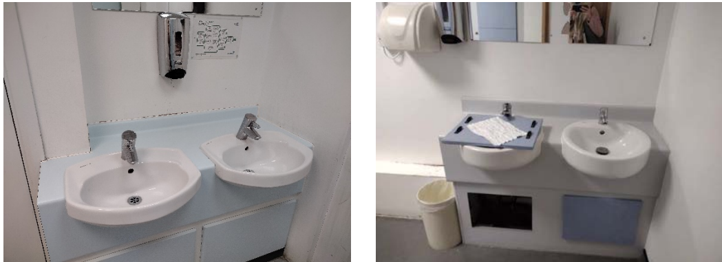
Figure 6: Examples of water mixing taps
