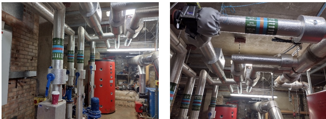
Figure 5: Examples of heating pipes insulation
