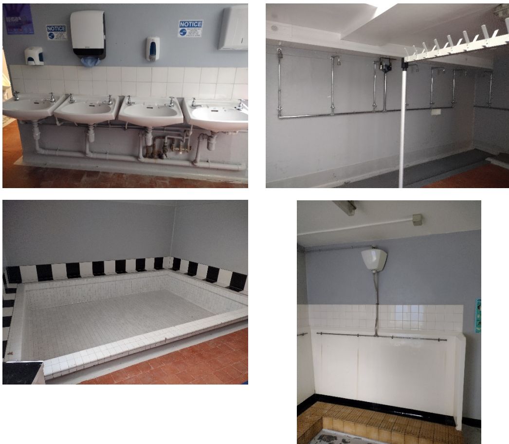
Figure 11: Examples of water equipment in East Block
